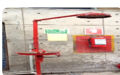
Eye Wash Station
